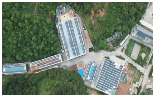
Ducheng Roof Solar Power Station
