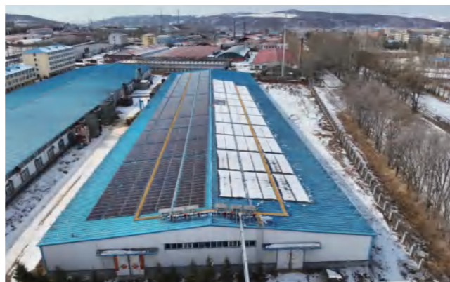
Mulingke Roof Solar Power Station
