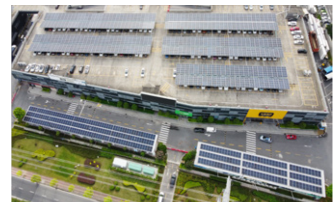
Our Choice Rooftop Solar Power Station
