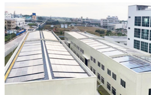
Baoying Rooftop Solar Power Station
