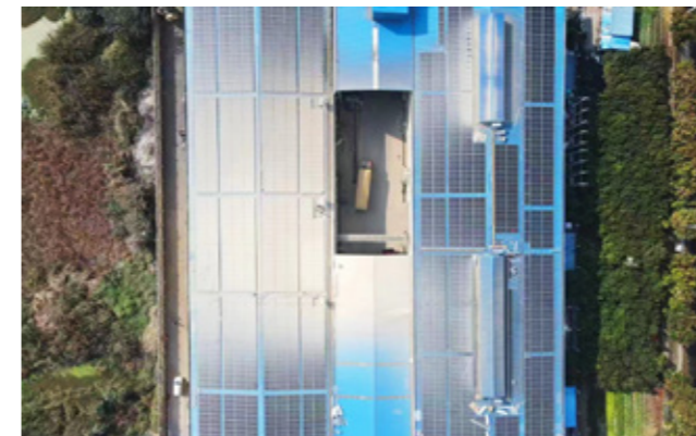
Tianfeng Rooftop Solar Power Station
