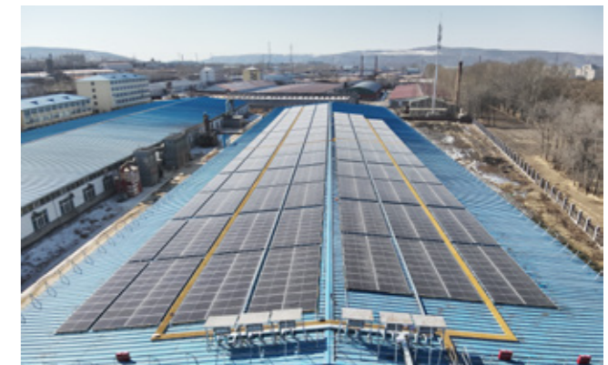
Muling Rooftop Solar Power Station
