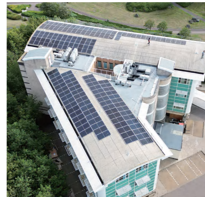
UK MANAGEMENT COLLEGE Solar Power Station
