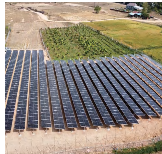
Snowflake Ice Factory Solar Power Station
