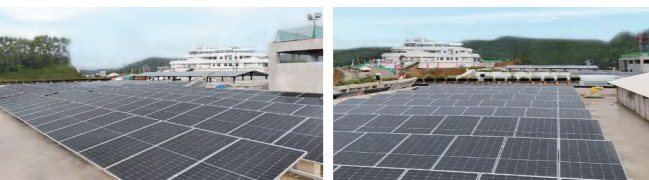
Rooftop Power Station Built in Indonesia's New Capital
