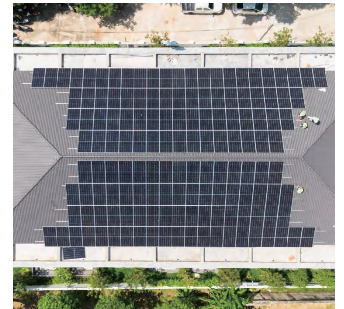
CS International Rooftop Solar Power Station
