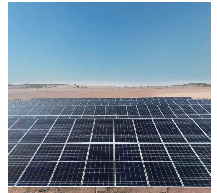
Solar Pumping Power Station
