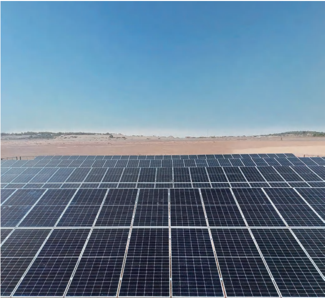
Solar Pumping Power Station
