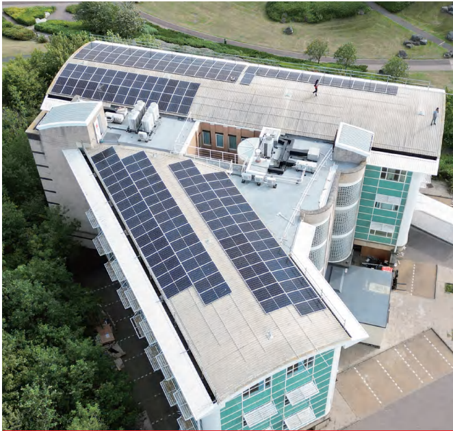
UK MANAGEMENT COLLEGE Solar Power Station
