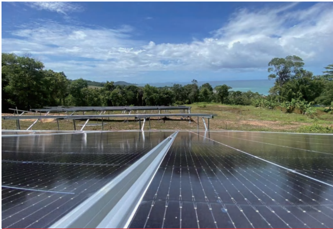
New Community Concentrated Solar Power Generation System
