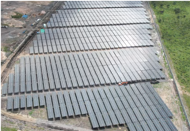
KEDA Ceramics Solar Power Station
