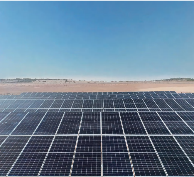
Solar Pumping Power Station
