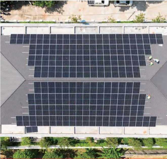
CS International Rooftop Solar Power Station
