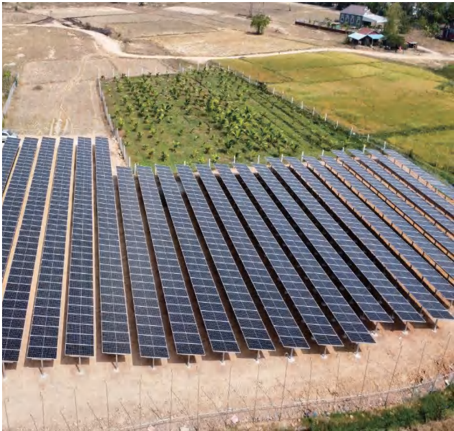
Snowflake Ice Factory Solar Power Station
