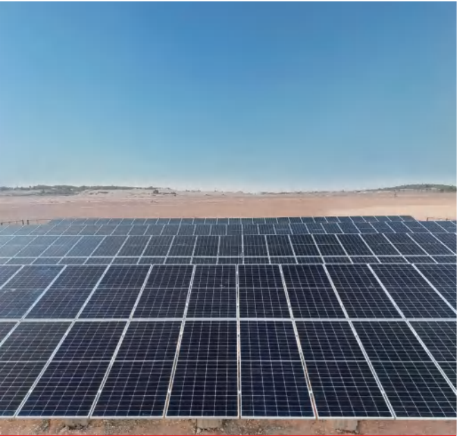
Solar Pumping Power Station
