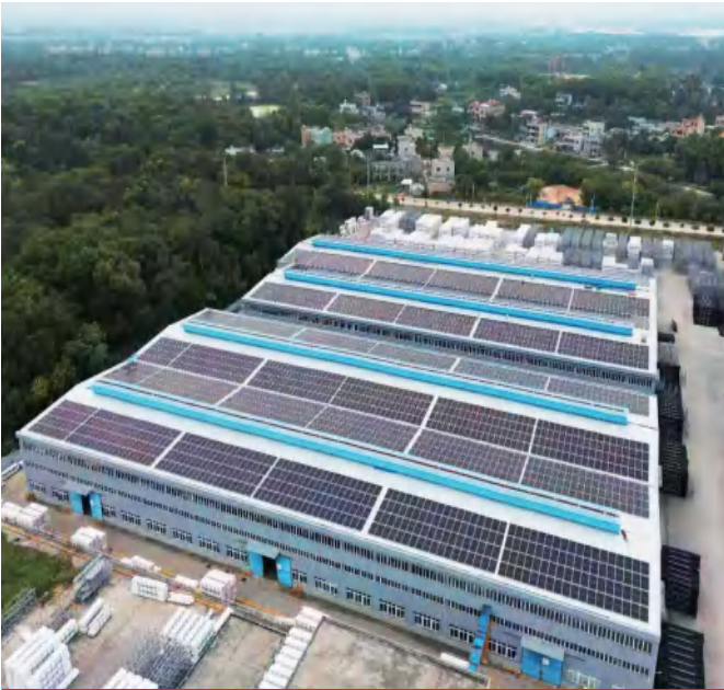
Dingan Roof Solar Power Station
